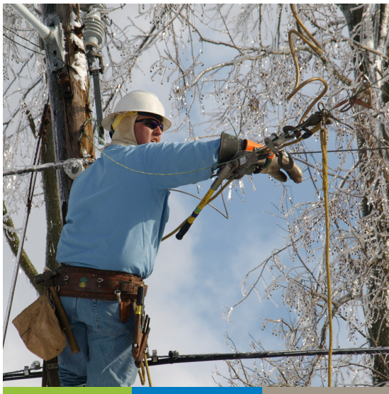
A line technician working in the harsh conditions of the 2021 ice storm.
