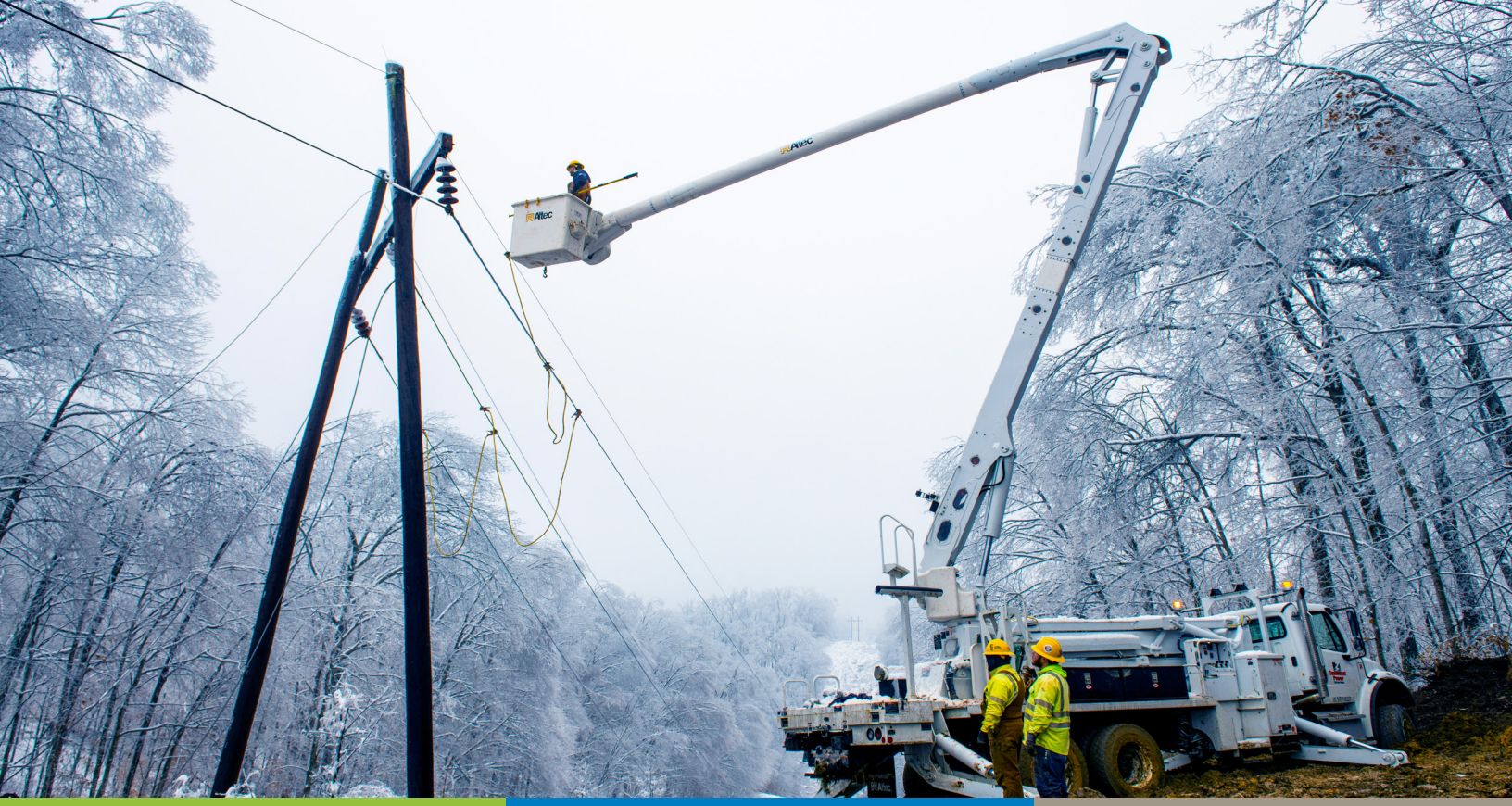
February 2021 ice storm caused significant power outages across the state.
