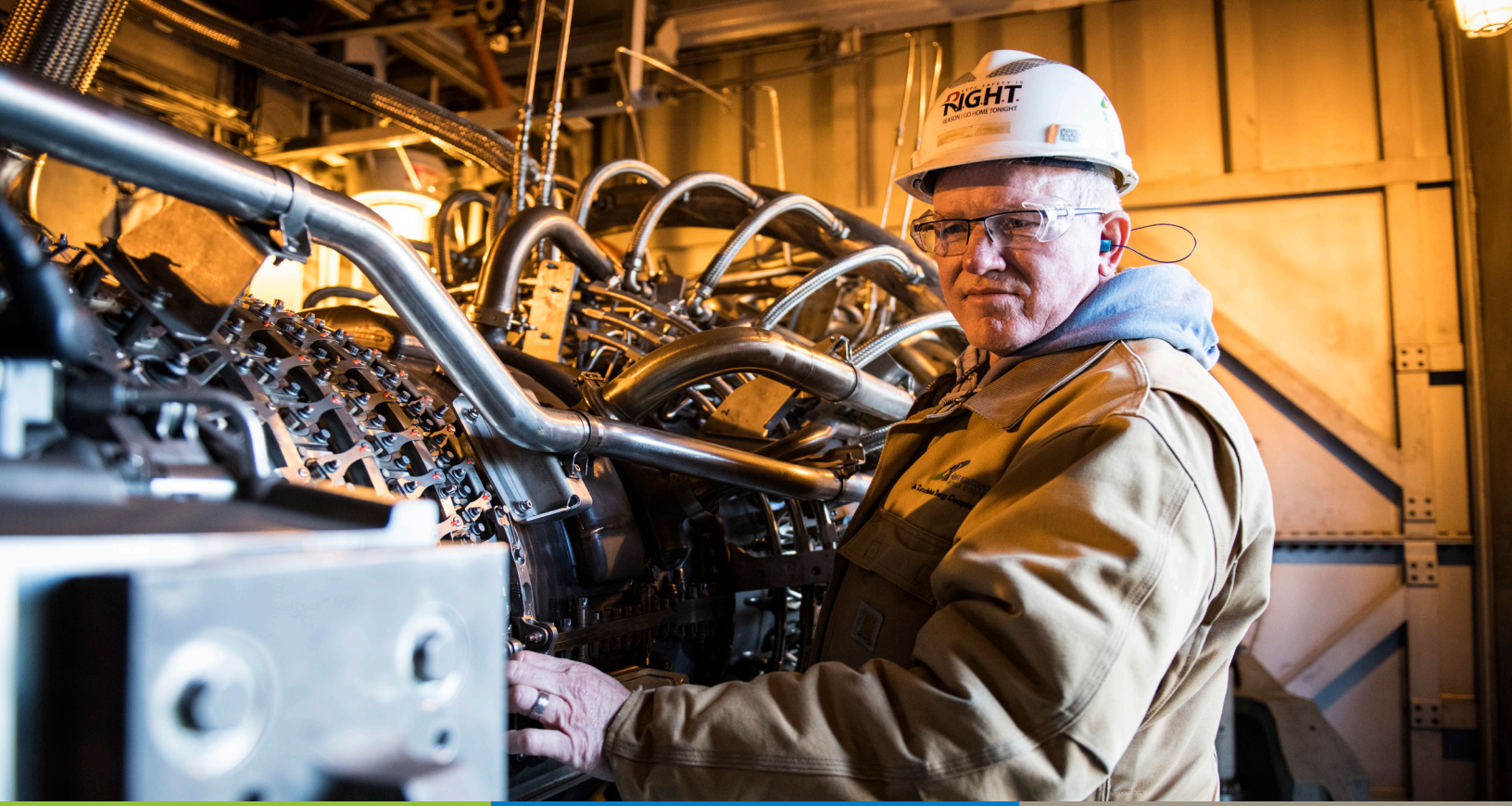
Smith Station overhauled one of its turbines in 2021.
