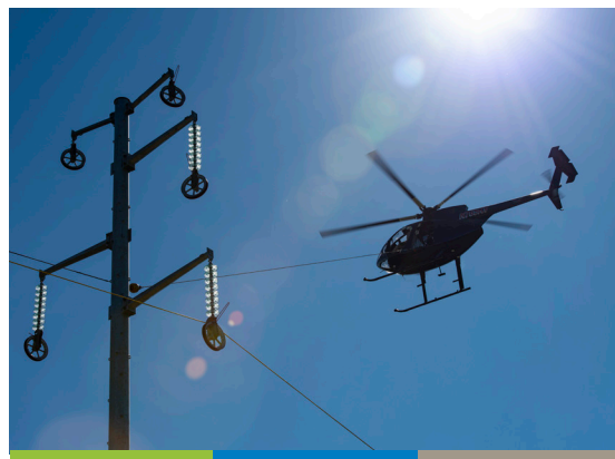
EKPC team members use a helicopter to pull a conductor in place over two miles in Broughtontown.
