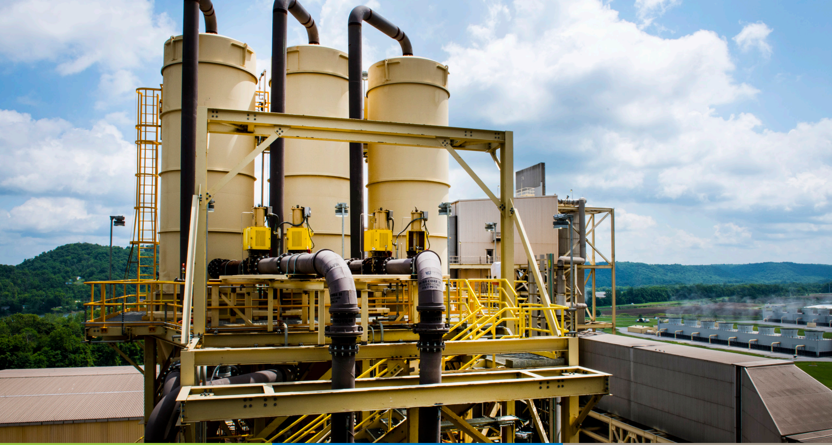
Spurlock's new cooling tower is a significant upgrade from previous infrastructure.
